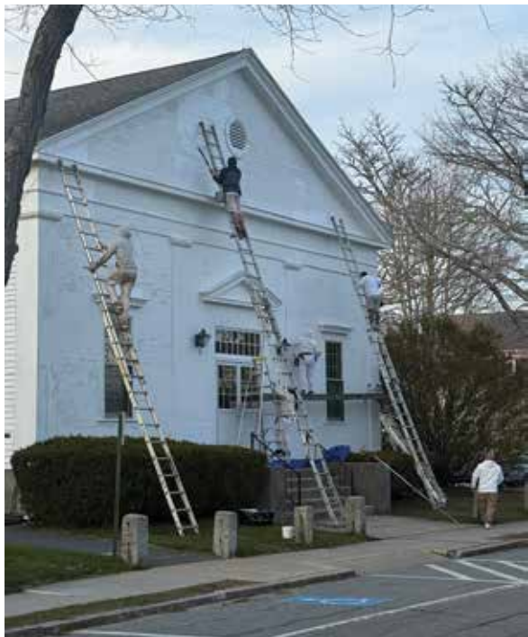
The Mattapoisett Congregational Church was getting a new coat of paint on Tuesday evening. It was finally a day with some great weather. Photo by Sam Bishop
